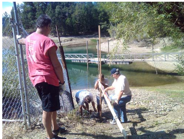
Wayne, Bryant, Hugh and Buzz planning the stair forms for the dinghy dock
